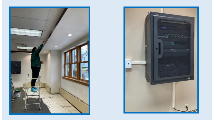
Right: A new paint job Left: The sound system box
